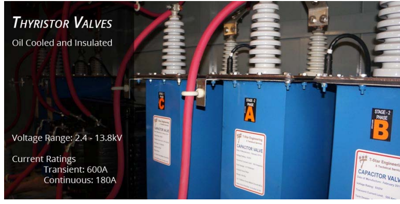
Figure 1. Thyristor Valves—By T-Star Engineering and Technical Services
