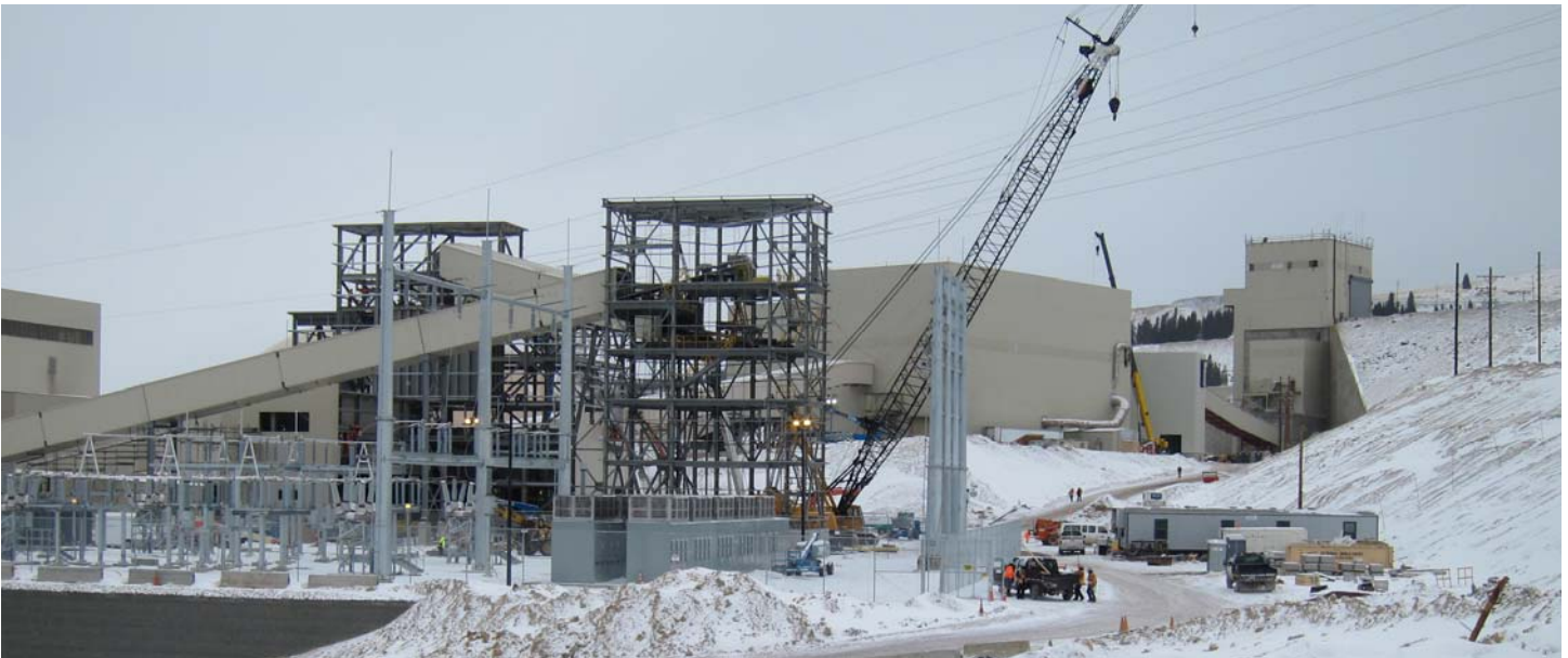
Two 19 MVAR 5-stage metal-enclosed harmonic filter banks located at the Climax molybdenum mine in Climax Colorado, United States. This project required derating due to its extreme altitude (3462 meters, or 11,360 feet above sea level).
