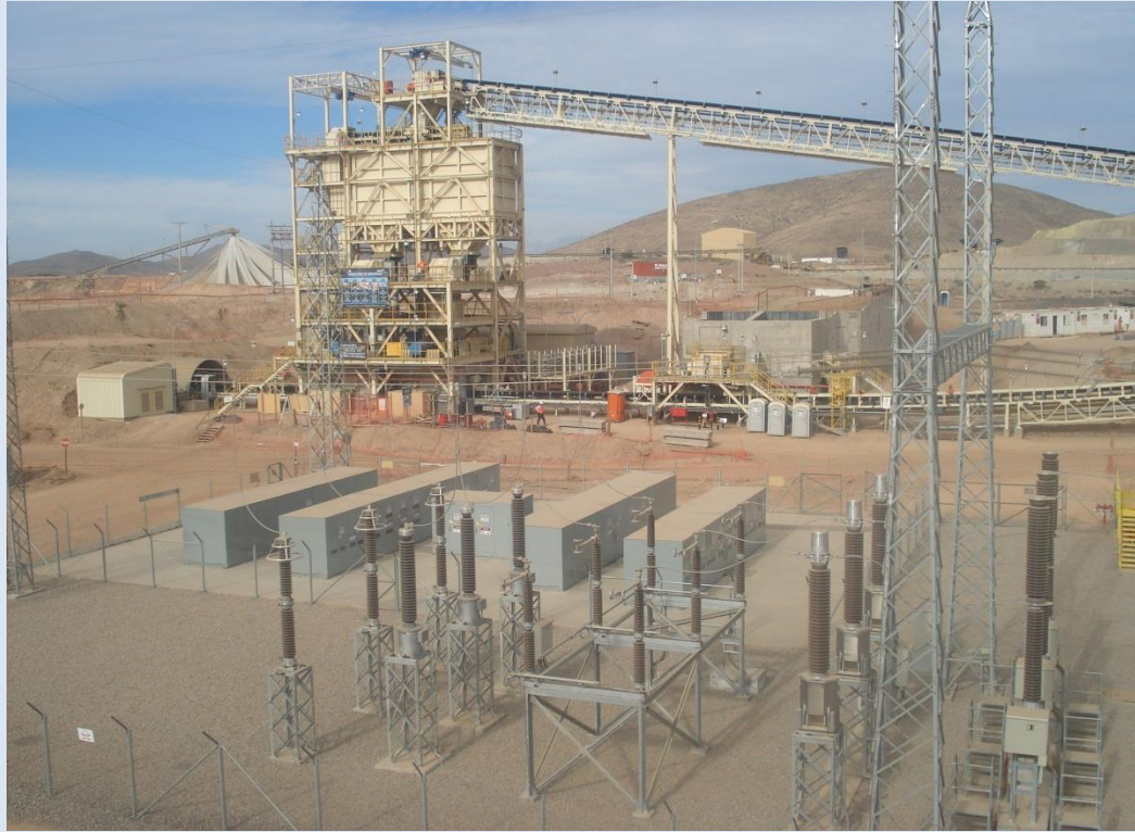
Typical Harmonic Filter System installed at a remote mine at 10,000' in South America. This system consisted of three large multi-tuned harmonic filter banks. Enclosures were built with low profile design to allow for shipment in high-cube containers.
