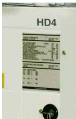
The nameplate, located on the front panel, enables all the circuit-breaker characteristics to be identified.
